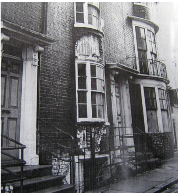
9 | Photo by Brighton Borough Surveyor showing dilapidations. Image courtesy of the Royal Pavilion, Libraries and Museums, Brighton and Hove
